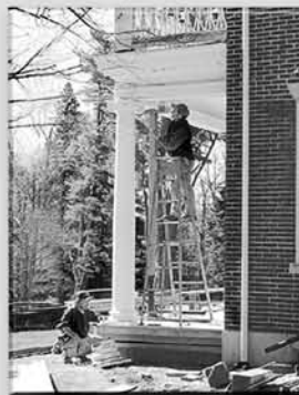
Nelson Emerton and Mike Klenowski carefully install the new columns on Woodlawn's front portico
