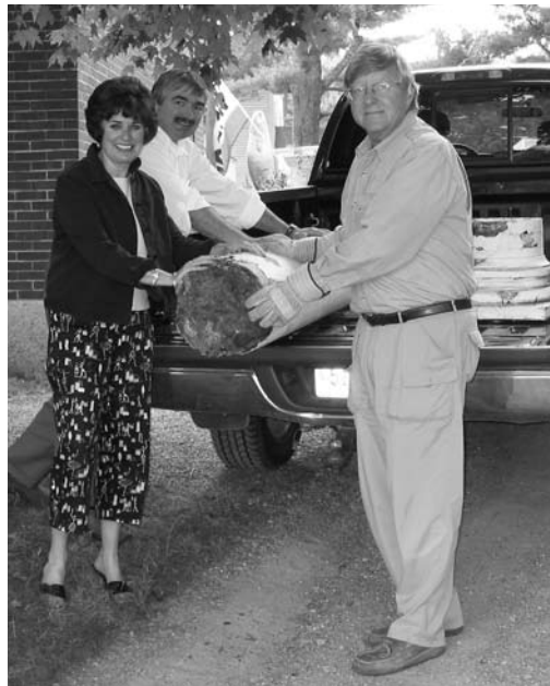
Trustees Jeffrey Dow, Jacqueline Dearborn, and Gregg Hannah help remove one of the badly deteriorated front columns.
